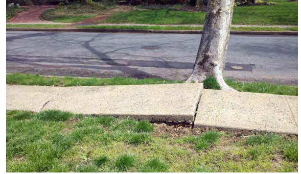
Potential environmental hazard: Questionable sidewalk
